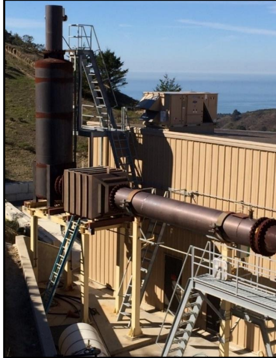
Figure 17. View of Exhaust System of the One Unit
