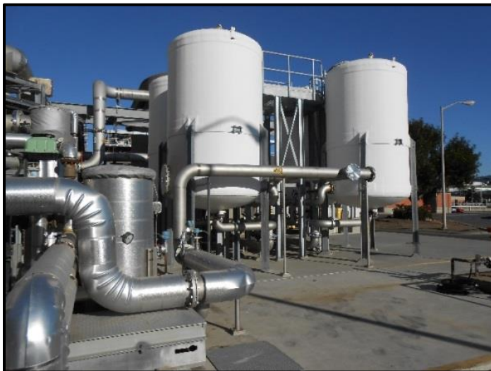
Figure 14. Siloxane Canisters at East Bay MUD
