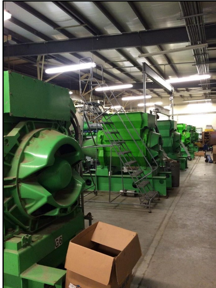
Figure 16. View of Engines from the Generator-End
