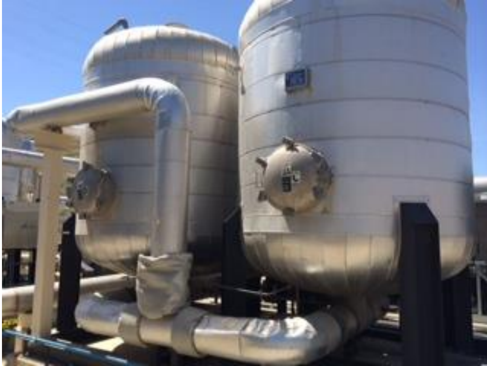
Figure 23. General Setup of Vessels for the Siloxane Removal System (Four vessels are incorporated into the system)
