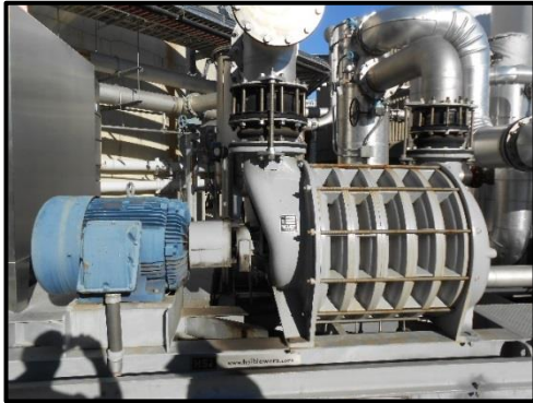
Figure.13. Biogas Compressor at East Bay MUD
