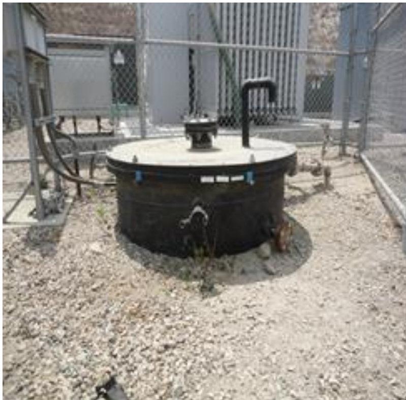
Figure 26. V-120 Condensate Holding Tank
