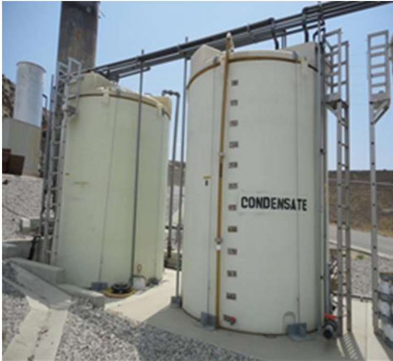
Figure 25. V-101A Separator Tank
