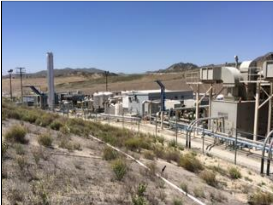
Figure 22. Overview of Chiquita Canyon Power Generation Facility
