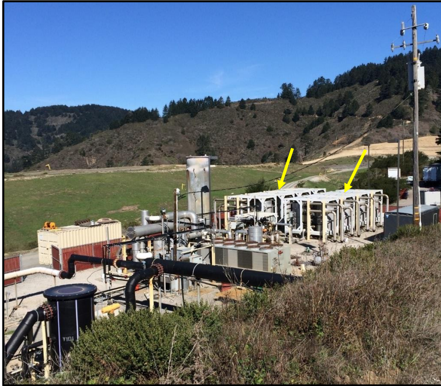
Figure 18. Overview of a Portion of the Gas Treatment System (arrows indicate the two eight-canister banks)
