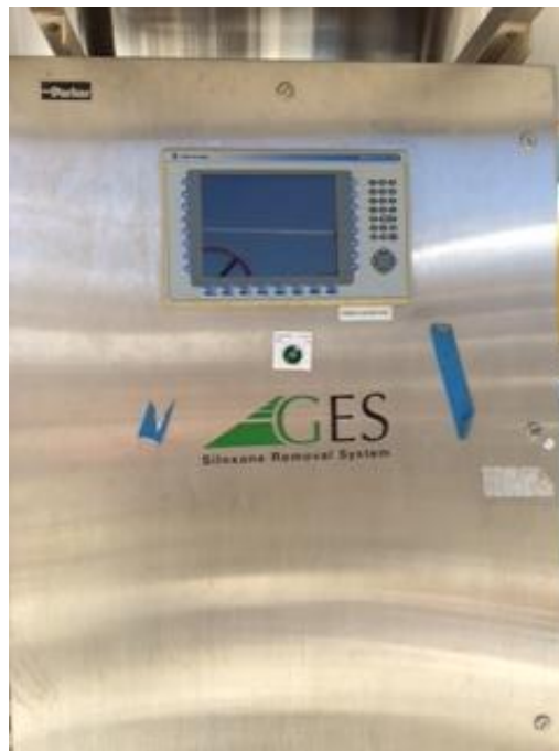
Figure 24. Parker Siloxane Removal System Control Panel
