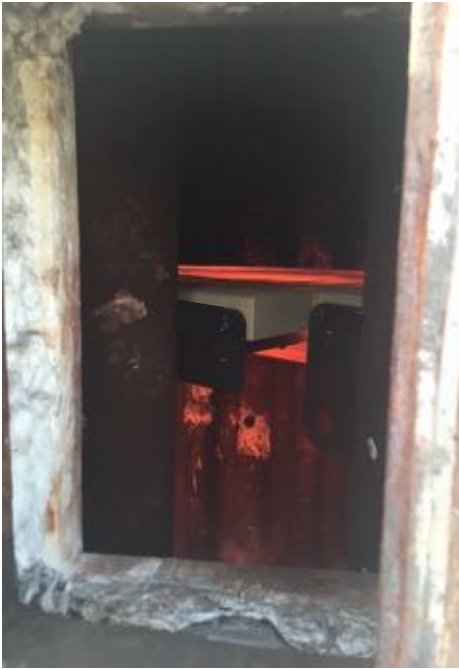
Furnace side port
