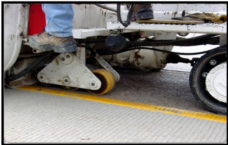
Figure 2-6: Slurry Recovery Vacuum on Texture Planer
