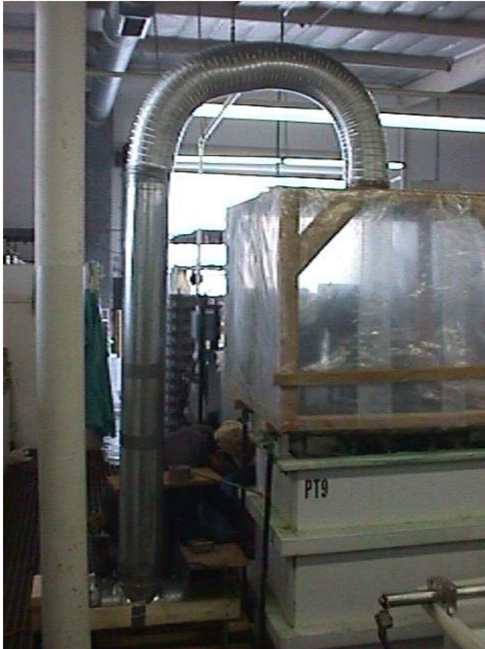
Figure 3 – Photo of Temporary Ventilation System
