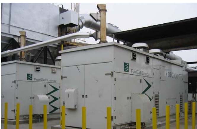
Figure 11: 250 kW Fuel Cell Unit
