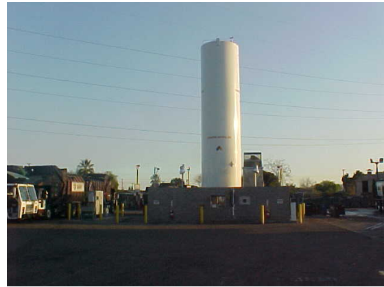
LNG Fuel Station and Storage Tank
