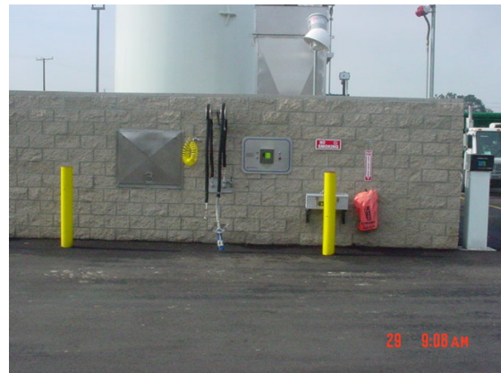
LNG Station Control Panel and Dispenser
