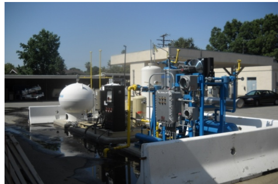
CNG Station Full View
