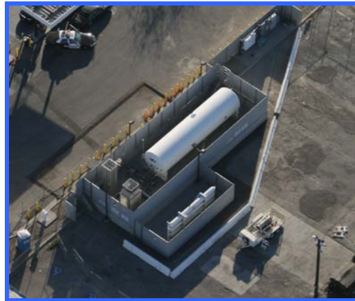
Figure 1: East Valley Regional Fueling Facility
