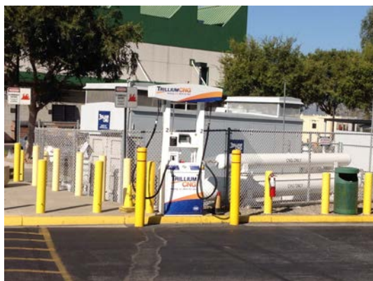
Figure 1: Public Access CNG, SCAQMD Headquarters, Diamond Bar, CA
