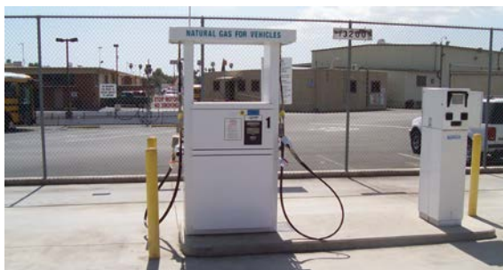
Figure 1: Public Access Fueling Station
