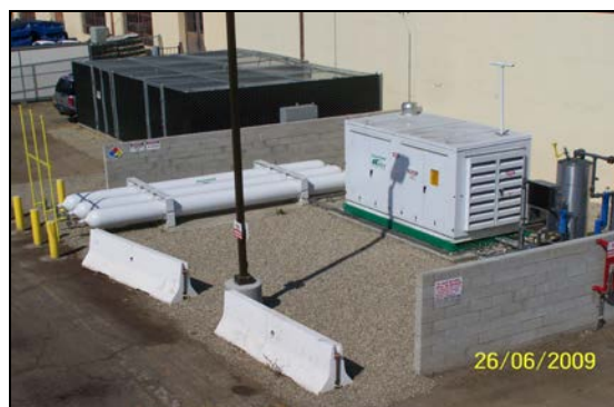
Figure 1: CNG Station Filter Dryer & Compressor at City Yard
