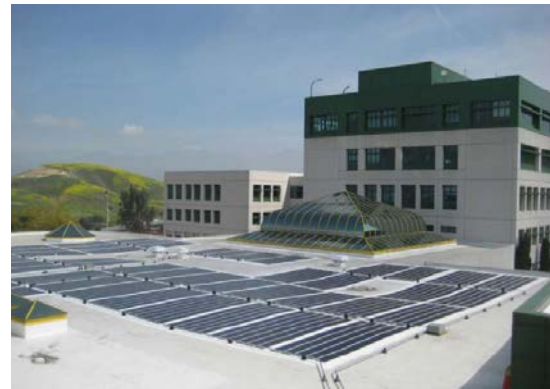
Solar Roof Panels on SCAQMD Building
