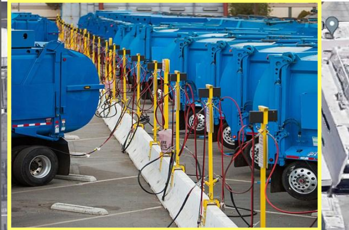
Simultaneous Time Fill System (Common Refuel Method for CNG fleet trucks)
