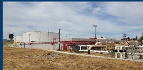
Pipeline and additional 3M gallons storage capacity became operational October 2019
