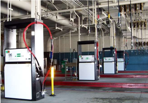
Figure 1: Single-Hose CNG Dispensers
