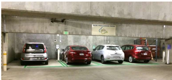
Figure 3: Getty Center parking structure, Level 2 EVSE
