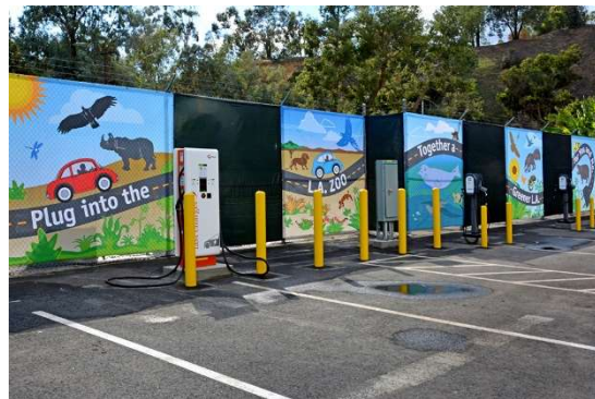
Figure 1: Los Angeles Zoo, DC Fast Charger and Level 2 EVSE (electric vehicle supply equipment)
