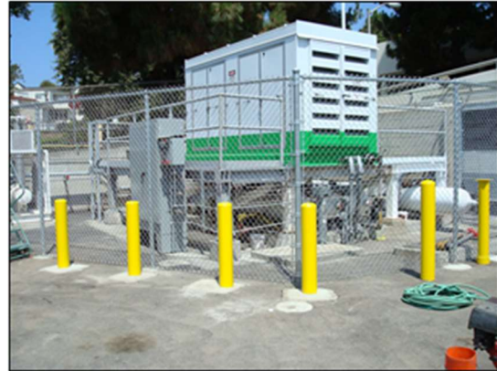
Figure 1: Compressor with Catwalk
