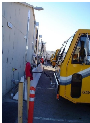
Figure 2: Time Fill Posts
