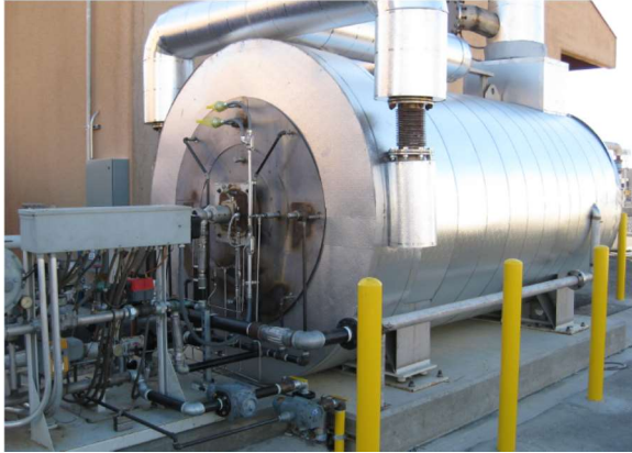
Figure 1: TVRWRF Noxtech® Reactor
