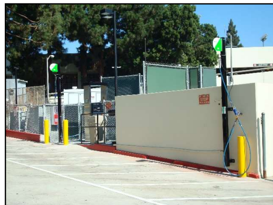
Figure 2: Station Fueling Ports
