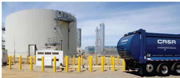
Figure 16: CR&R's Anaerobic Digester
