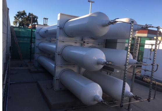
Figure 1: CNG “Cascading” Storage Tanks
