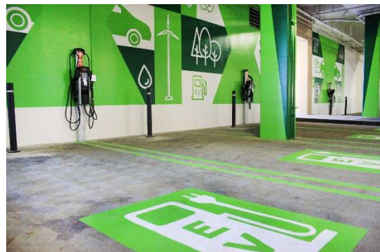
Figure 1: EV Charging Stations: Westfield Santa Anita Mall, Arcadia
