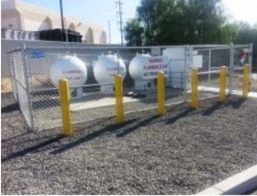
Figure 2: CNG Storage Vessels
