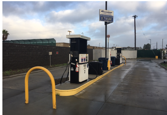
Figure 2: Public CNG Station
