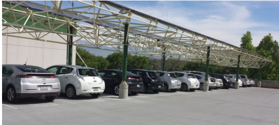
Figure 3. Level 2 EV Chargers Under the Solar Carport in the Upper Parking Lot Near the Employee Entrance
