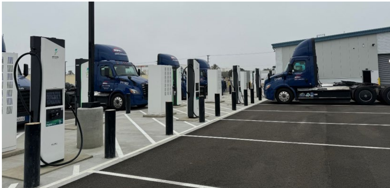
Figure 9: Partial Deployment of NFI Daimler Class 8 BETs and Charging Infrastructure
