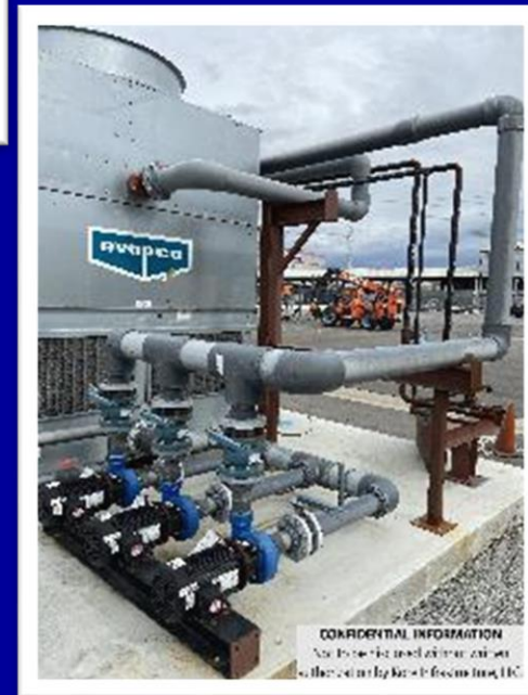
Cooling Tower, Pumps, Piping in place
