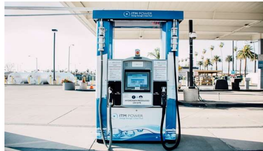
Figure 1: Installed Dispenser at Site
