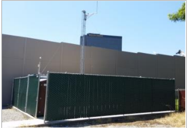
Looking at the probe from the East.
