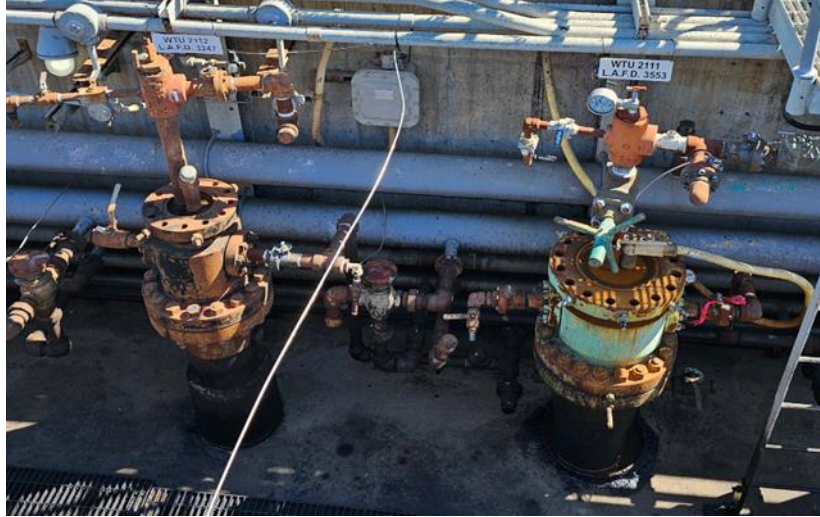
Figure 1.2 – Example of Wellheads Inside a Well Cellar
