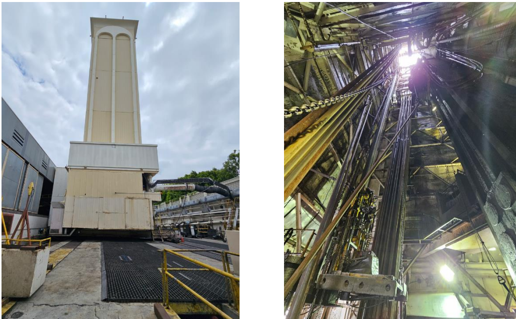
Figure 2.11 – Photo on left shows electrified drilling/workover rig and photo on right shows inside view. Note that this drilling/workover rig is on a rail and can only be used at this specific site
