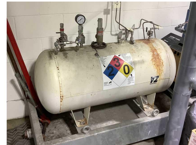
Mercaptan storage tank
