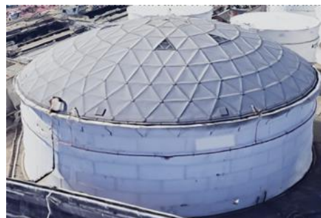
Figure 2-1- Domed Storage Tanks
