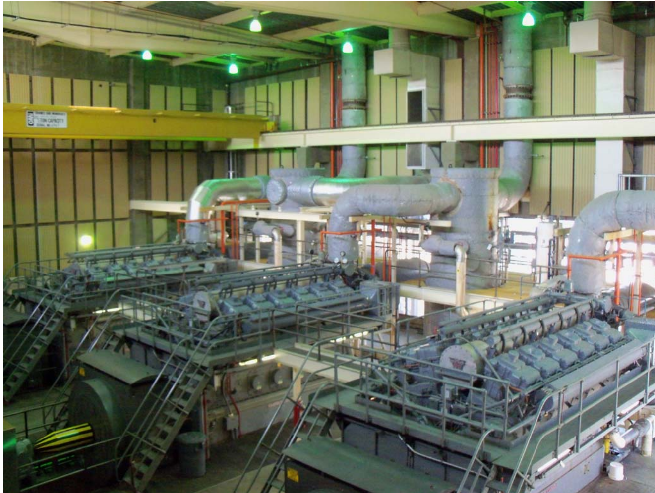
Figure 2-1: Plant 1 Engines 1, 2, and 3 (pictured left to right)
