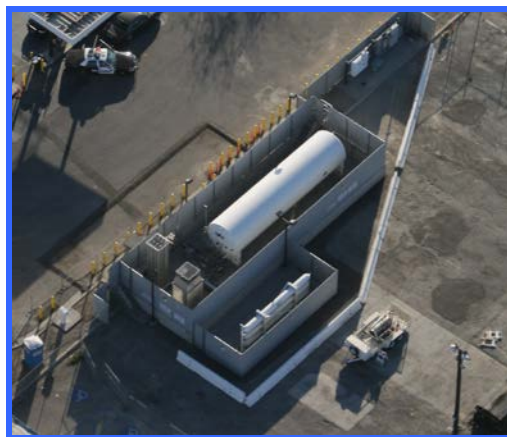
Figure 1: East Valley Regional Fueling Facility
