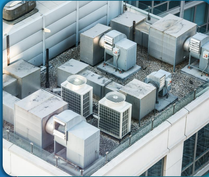
Commercial Combustion Water/Space/Heating/ Cooking/Others
