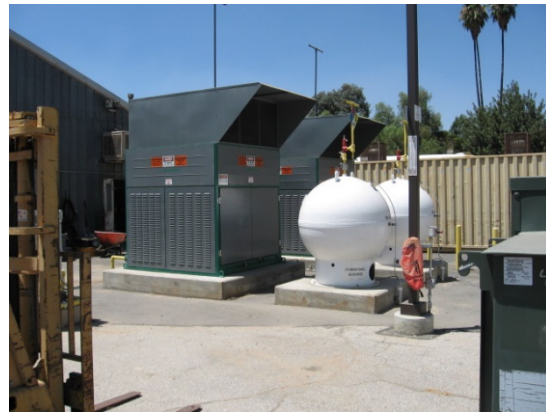
Figure 1: Skid-Mounted Compressors and CNG Storage Spheres
