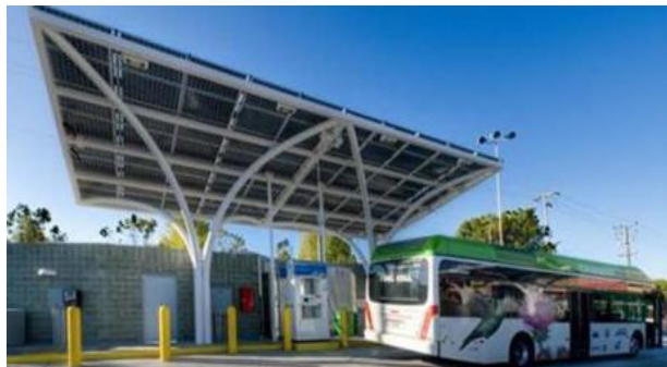
Figure 13: Transit Bus Hydrogen Fueling Station
