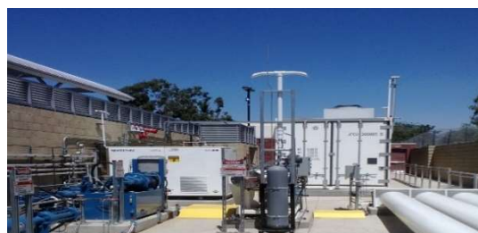
Figure 1: CSULA's H 2 Station interior (from left to right): high pressure compressors, H 2 chiller, 350 bar compressor, electrolyzer, 350 bar storage banks, visitor gallery
