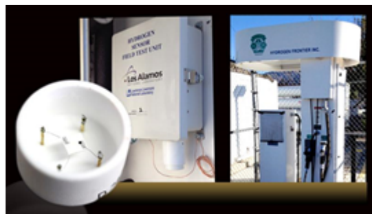
Figure 1: A close-up of a sensor element (left). Hydrogen sensor prototypes were installed at fueling station in Burbank (right) and Chino to assess their performance and long-term stability.
