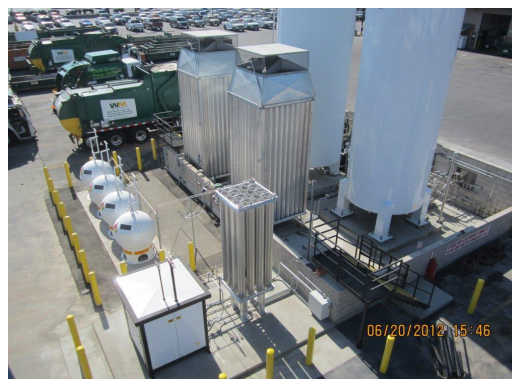
Figure 2: Rear View of Tank Installation and New Equipment and Components
