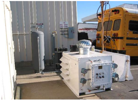
Figure 1: PYLUSD Bauer/P500 Compressor
