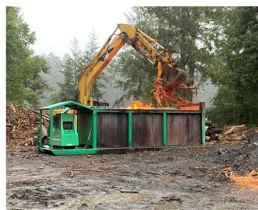
Figure 2-6 — Air Curtain Incinerator
