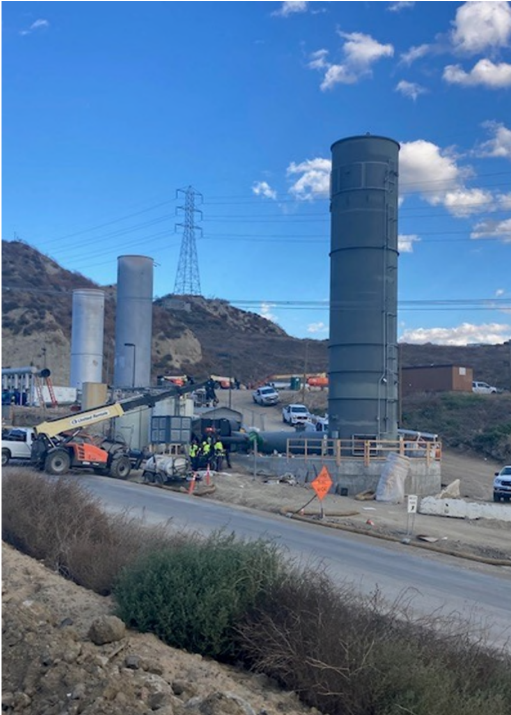
Figure 3. Picture of Chiquita's landfill gas flaring facility, showing the three existing flares.
