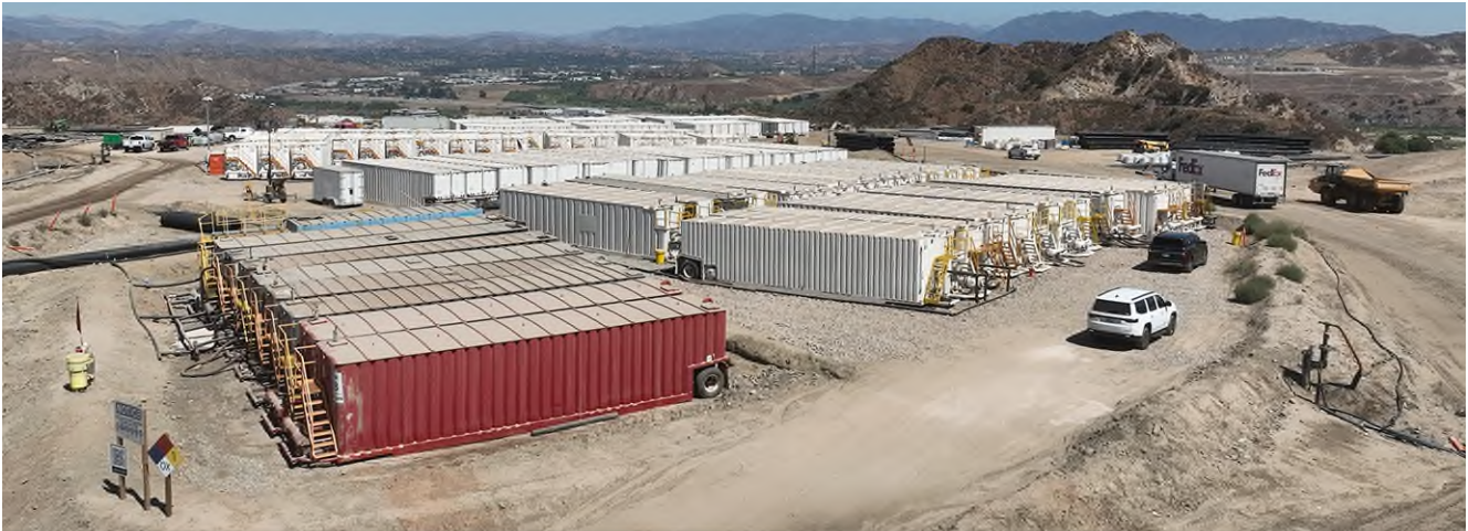
Figure 11. Images of a leachate tank farm at the Landfill.
