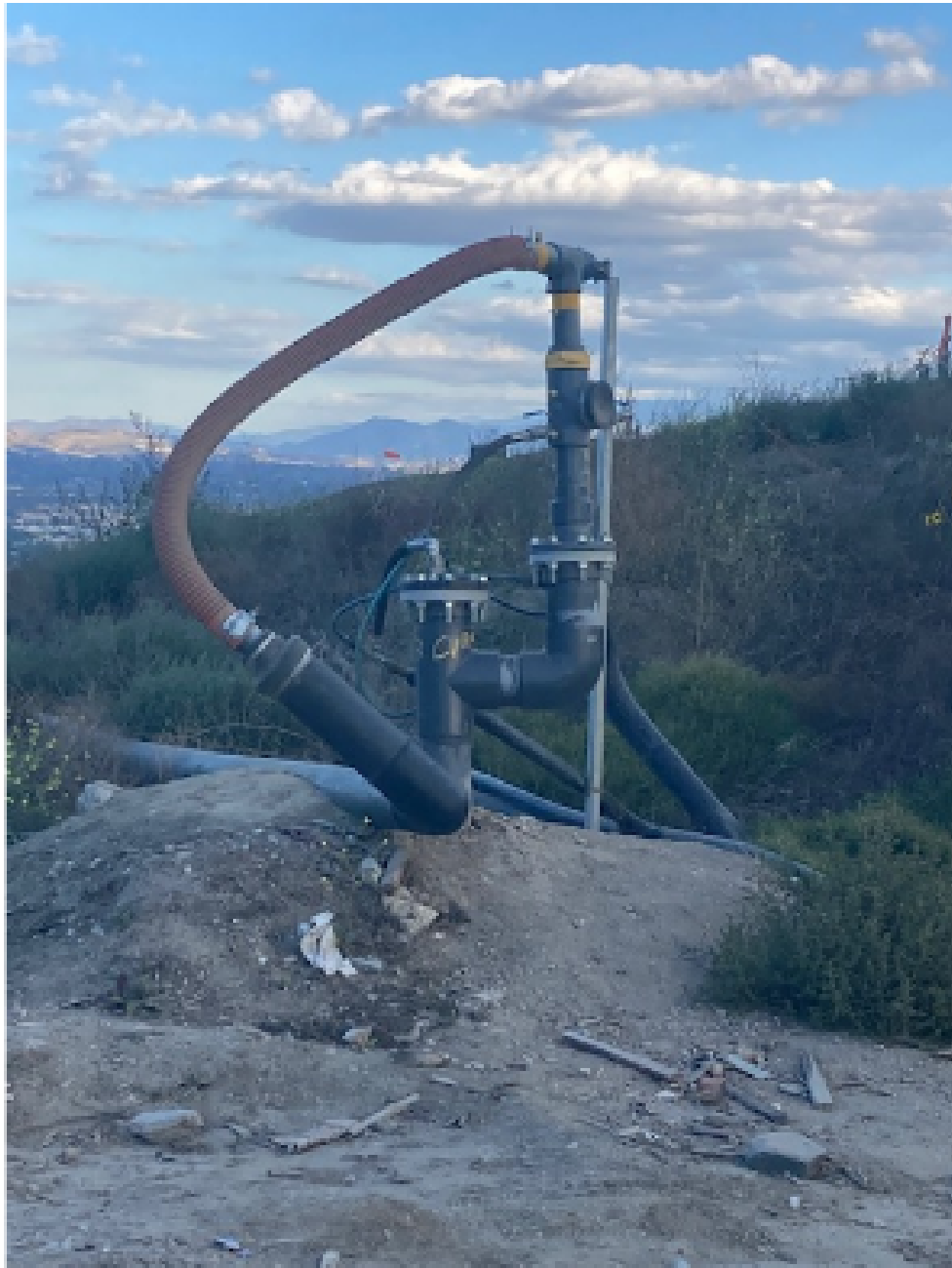
Figure 2. Picture of a vertical dual extraction landfill gas well. Chiquita installed over 220 such wells between December 6, 2023 and the end of October 2024.
