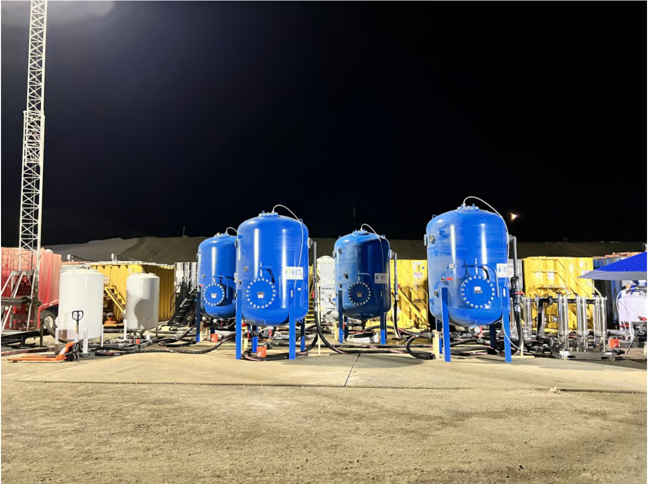
Figure 14. Picture of a GAC treatment system at the Landfill.
