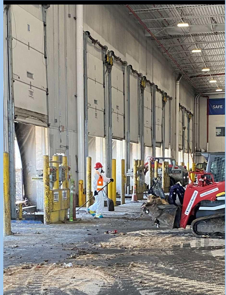
Photos taken by District staff August 4, 2026
