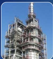
Process Heaters & Boilers
