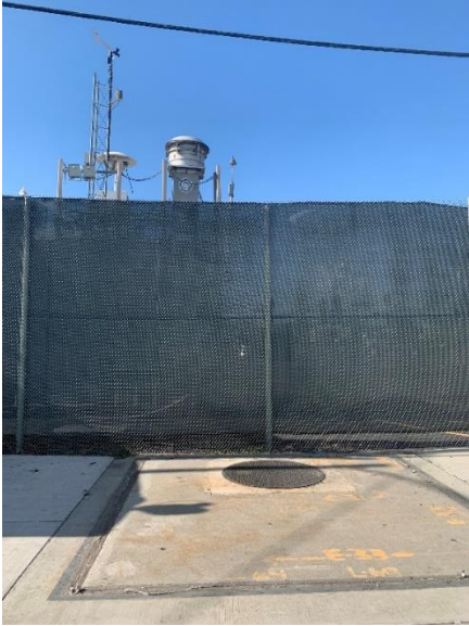
Figure 6 Manhole cover and inlet probe.
