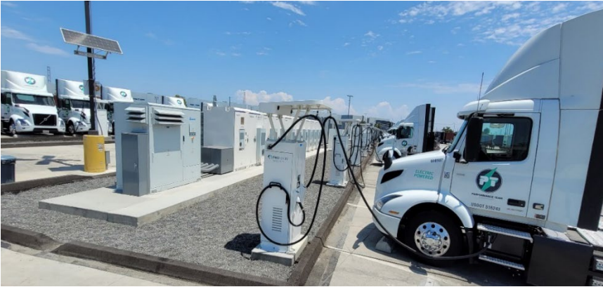
Figure 15: Class-8 EV truck charging at Denker Yard
