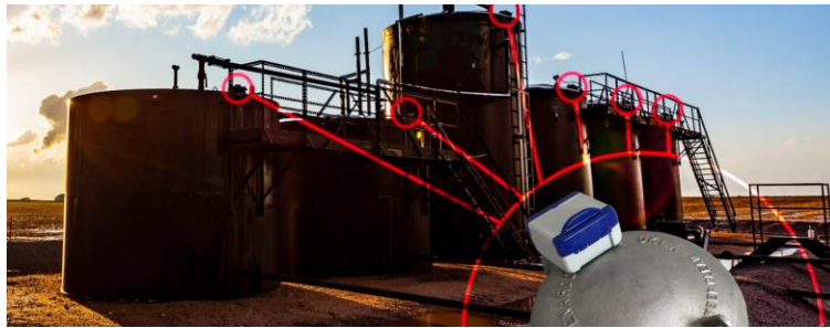
Figure 2.1 – Tank Battery at Oil Production Site
