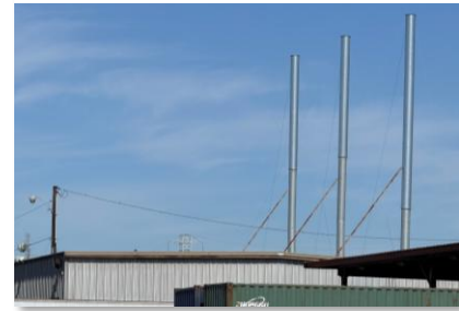
Figure 16 - Raised Exhaust Stacks
