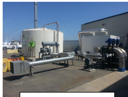
Figure 14 - Regenerative Control Equipment
