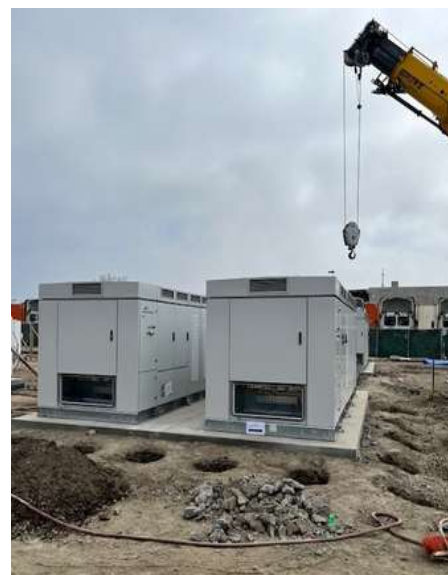
Figure 8: Schneider South El Monte Facility
