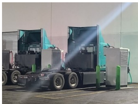
Figure 1. Switch-On Volvo VNR Electric trucks charging
